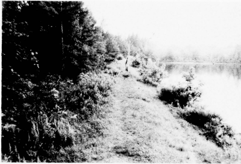
M. Maple Lake Dam — Upstream of Nesbitt Dam — View of Top of Dam Looking Towards Right Abutment
